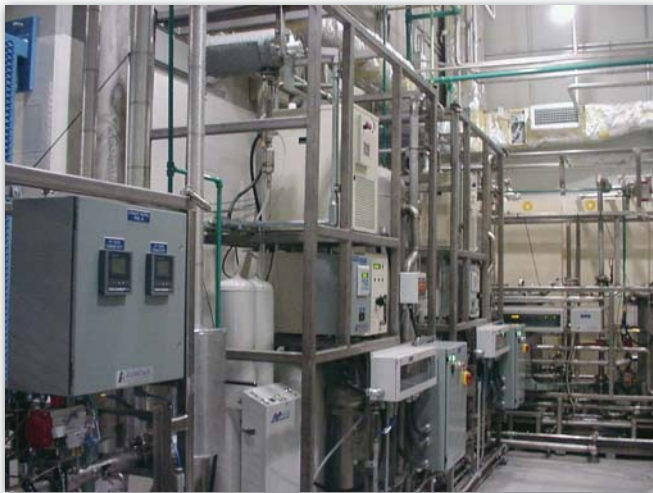
Modular Liquid Radwaste Systems
